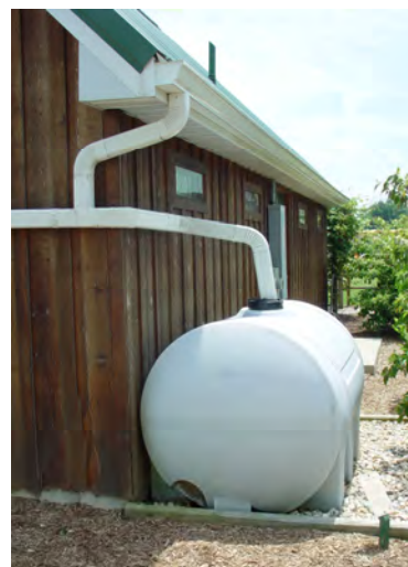
Cistern for harvesting stormwater that drains from the roof.
